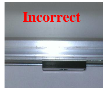
Figure 6: Improperly engaged lens and clip. Note: Lens extends below the top groove, and into the bottom groove of the aluminum channel
