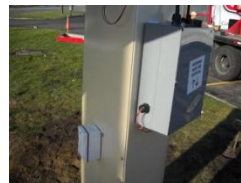
Radio on Sign at least 2.5' away from other antennas
